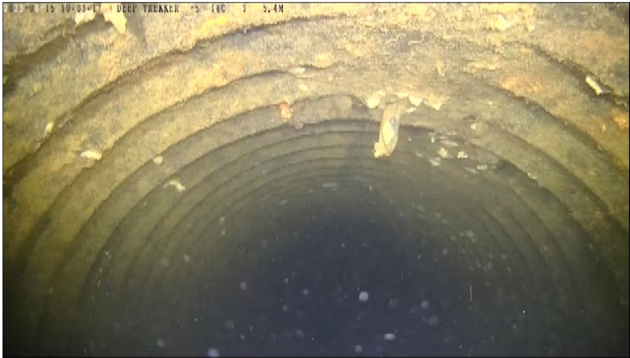
Photograph 4: Possible Pipe Puncture Observed at the Obvert (top) of the Duty Intake Pipe
