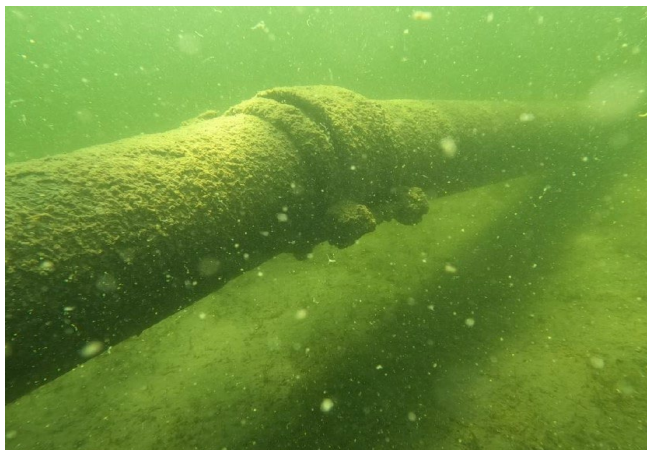
Photograph 1: Offset Joint in Emergency Intake Pipe
