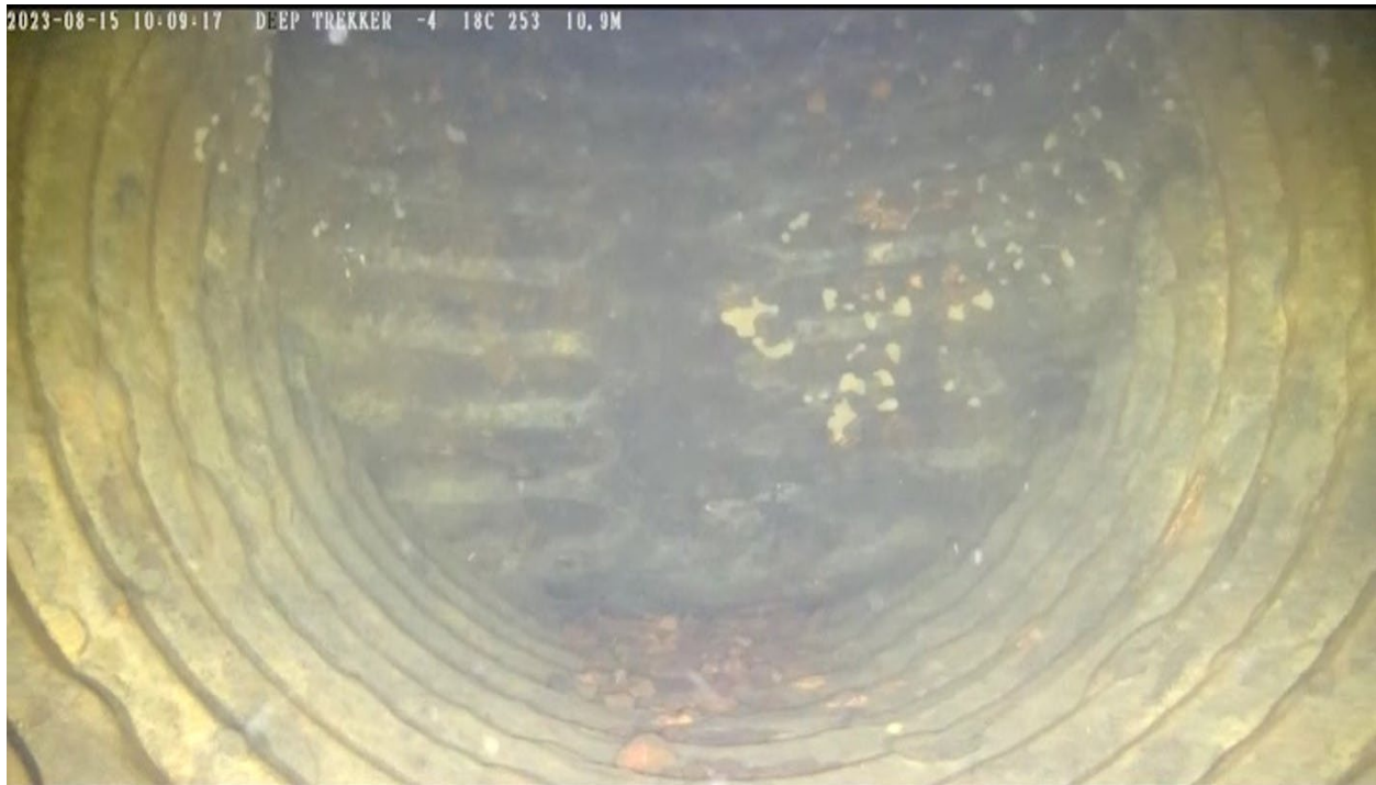
Photograph 6: Potential Dislodged Rust Particles at 90° Section of Duty Intake
