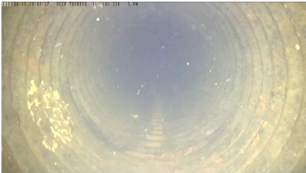
Photograph 3: Duty Intake Pipe – Minimal Sediment Along Invert
